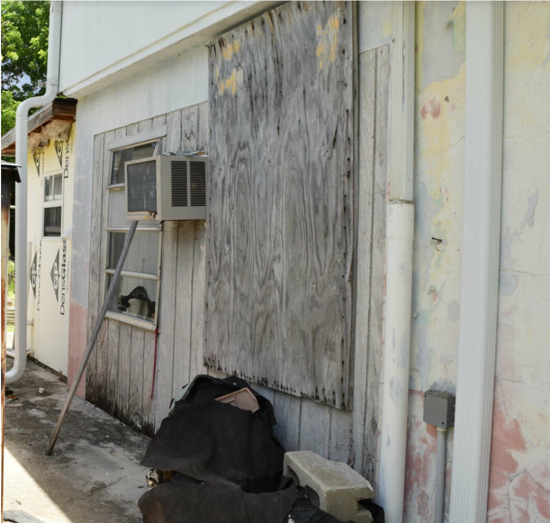
This image shows a section of Parchment's damaged roof and windows that have been earmarked for repairs. – Photo: Reshma Ragoonath
